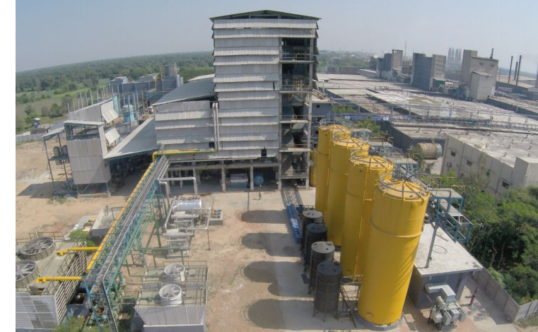
Multiple Effect Evaporator Plant (MEEP)
